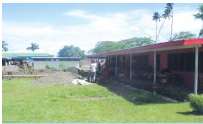
South Taveuni Secondary School. The existing school building on the right with a new 4 classroom building is being built to the left.
